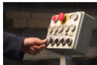
Each motor is started individually
